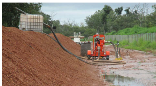
Basin overflow and pumping attempt, August 2018
